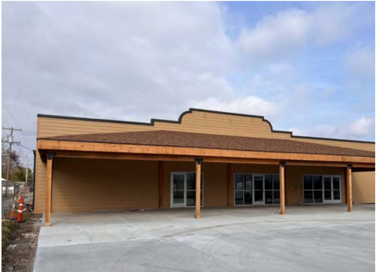
Prairie Sky Market currently under construction and scheduled to open January 2025. Photo by Madalyn Richardson.
